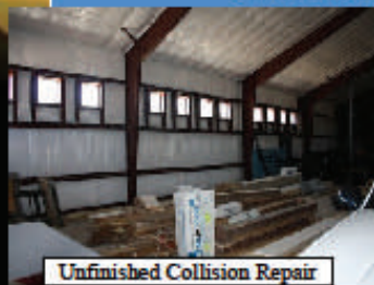
Unfinished Collision Repair
