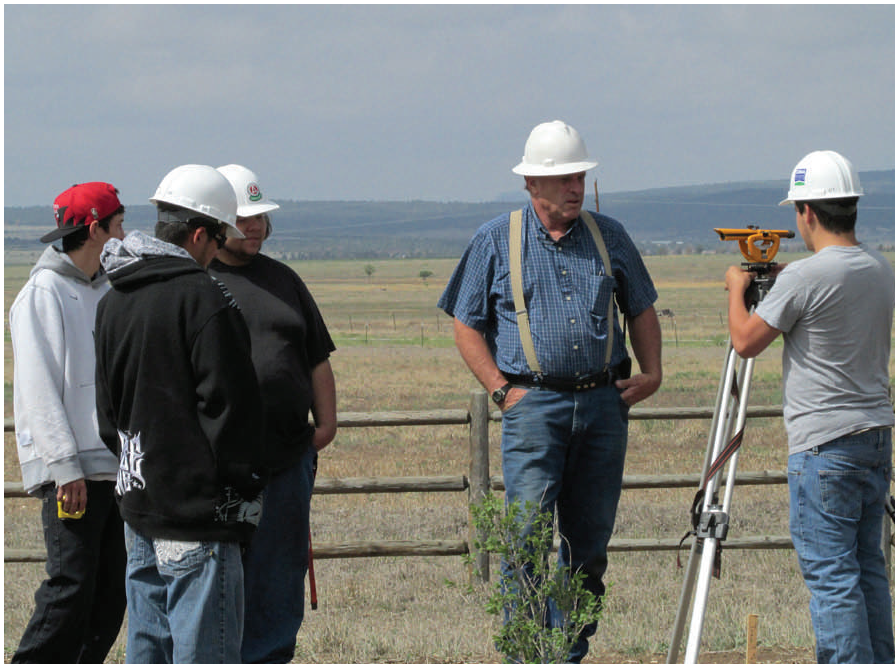
YouthBuild students receive guidance and direction from their Vocational Education Instructor Robert (Louie) Plagge on how to set up elevations to establish where bridges will be built at the Las Vegas National Wildlife Refuge.
