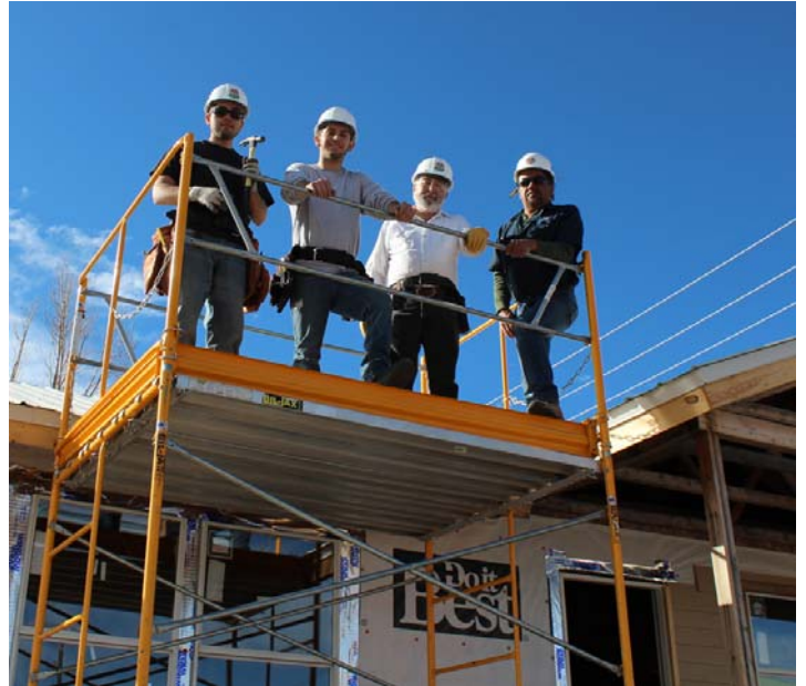
LCC students Jonathan Chavez, Jonathan Roybal, James Leger and LCC Building Technologies Instructor Joseph Montoya are installing a metal roofing system on a building technologies teaching module at the college.
