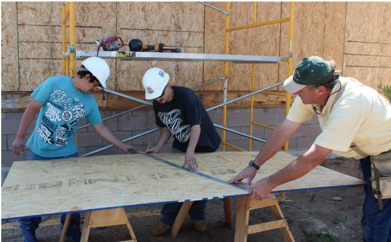
YouthBuild program participants work alongside their Vocational Education Instructor Robert (Louie) Plagge in scribing and cutting siding while at work on a model home on the LCC campus.
