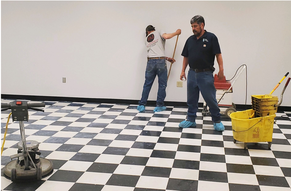
Luna's Joe Maestas works on applying a wax sealing to the floor of a cosmetology classroom. While the crew has focused on sanitizing and disinfecting buildings, it's also been an opportune time to take on other projects around campus.
